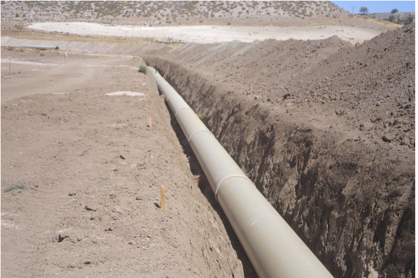
Pipeline of polyester reinforced with fibre glass.
